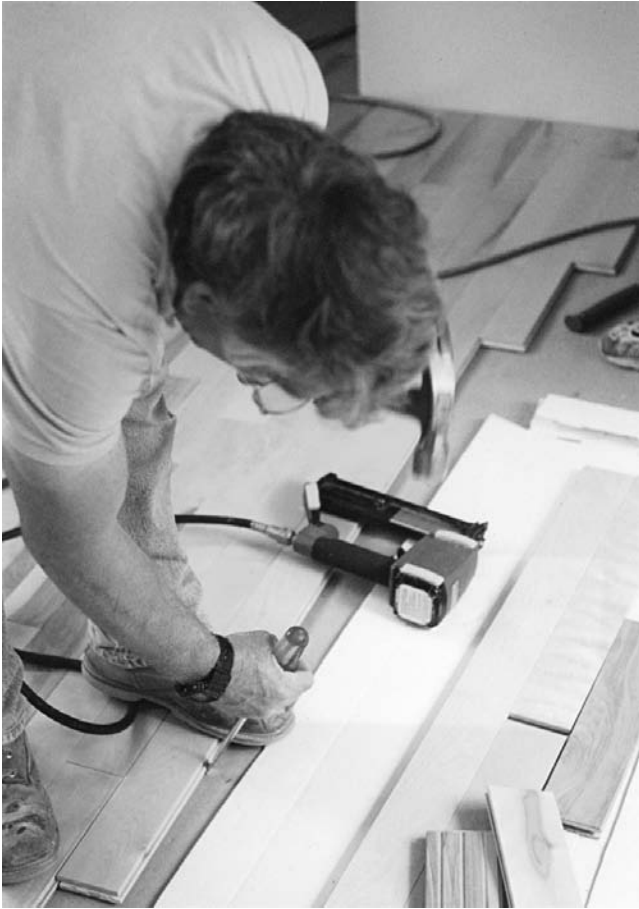
Figure 1-5 Self-advancement role: contractor; task: installing floor; activity: moving the wood into place.
